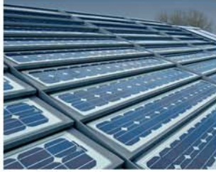
Photo-Voltaic roof system
